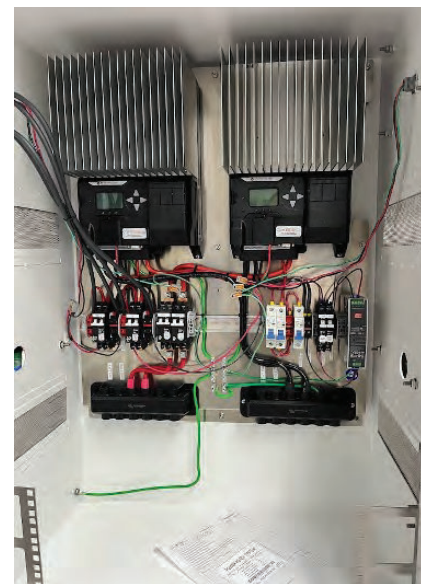
Inside of the controls cabinet
